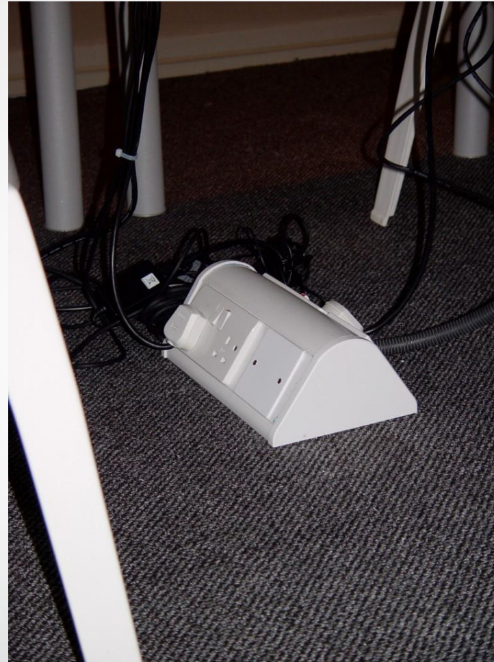
Cable floor box
