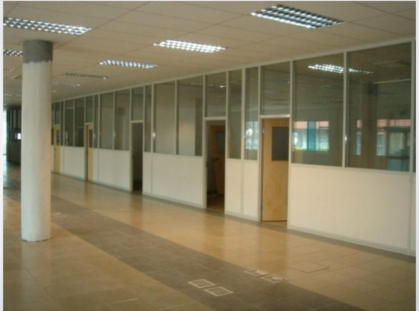
Framed glass partitioning
